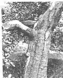
This fine old apple tree appeared to be past treatment, says Mr. Crane. Note how Davey experts, after cleaning out the decay, disinfecting and waterproofing, have braced the shell and filled it with sectional joints of concrete. This is an exclusive Davey process which allows for swaying and prevents cracking.
