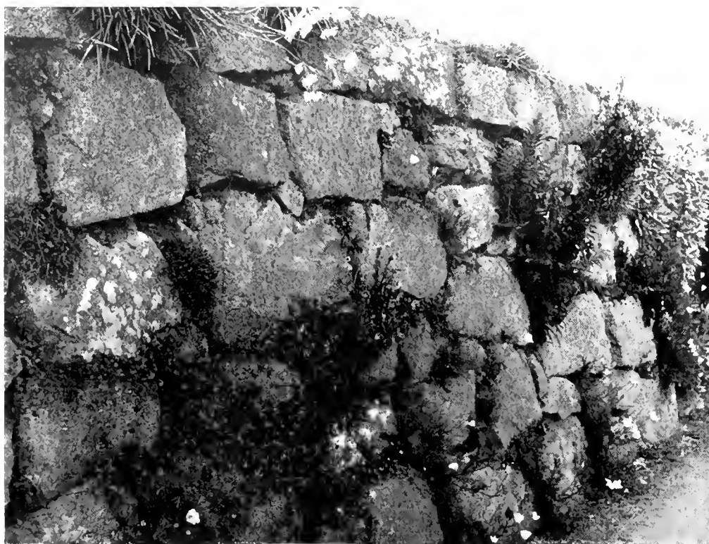
A DRY WALL, SHOWING IRREGULAR JOINTS FILLED WITH SOIL (NO MORTAR USED).
