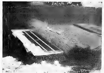
56. The best protection for a weak place. Old newspapers covering the joints
