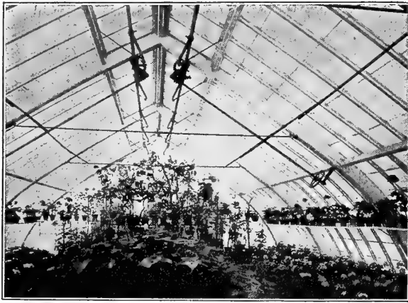
A Cypress Greenhouse owned by C. C. Converse, Malden, Mass. Lord & Burnham built it more than 30 years ago—it is still in prime condition. Made of CYPRESS, it is making a record for endurance that is fully worthy the marvelous qualities of "the Wood Eternal."
