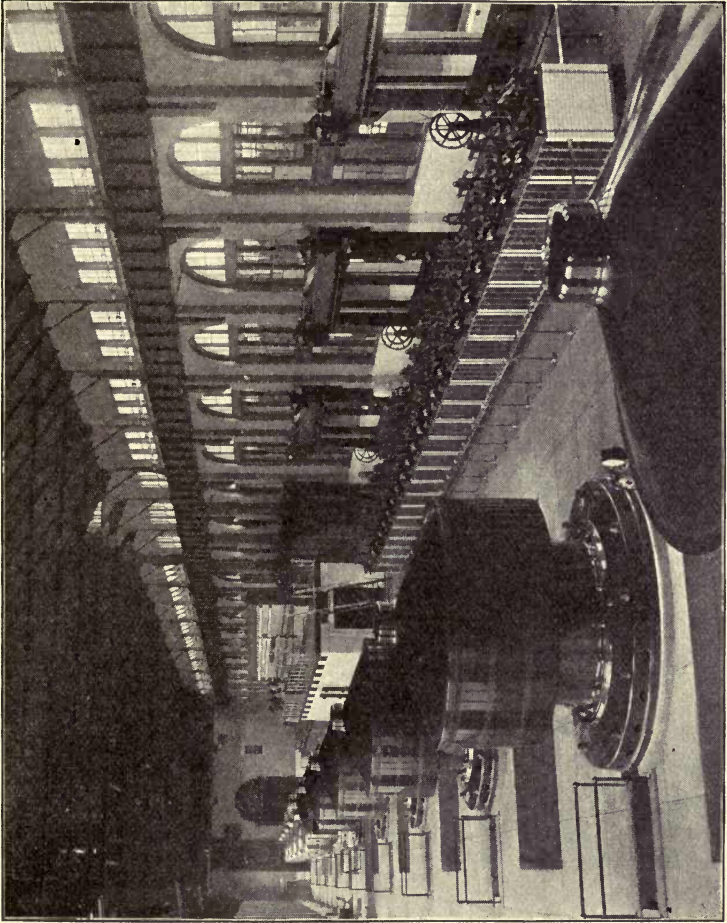
Interior of a Power House.
