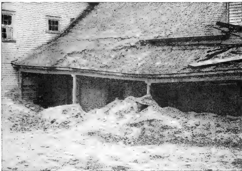
FIG. 298. — A roof collapsed by the weight of ash from Katmai, Alaska, one hundred miles distant. The drift in front of the porch is volcanic ash. ( National Geographic Magazine .)
