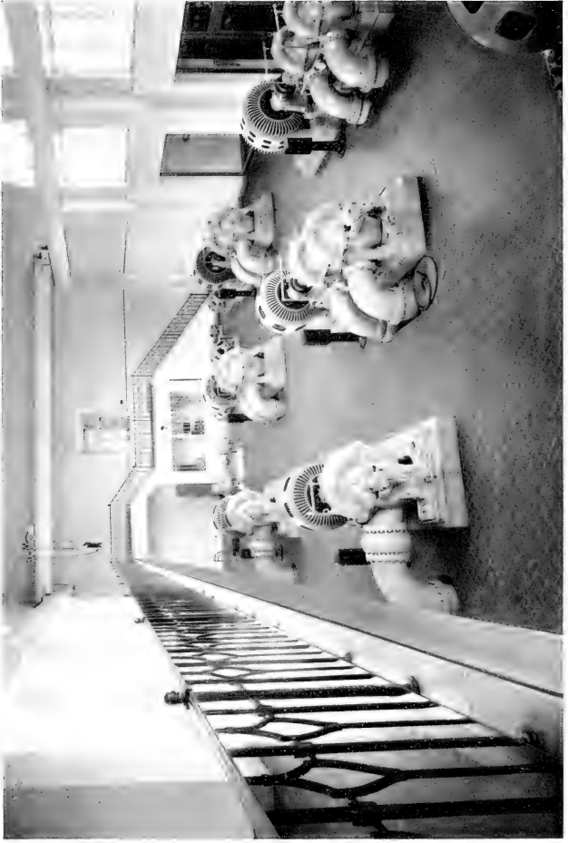
Washington electric pumping plant
