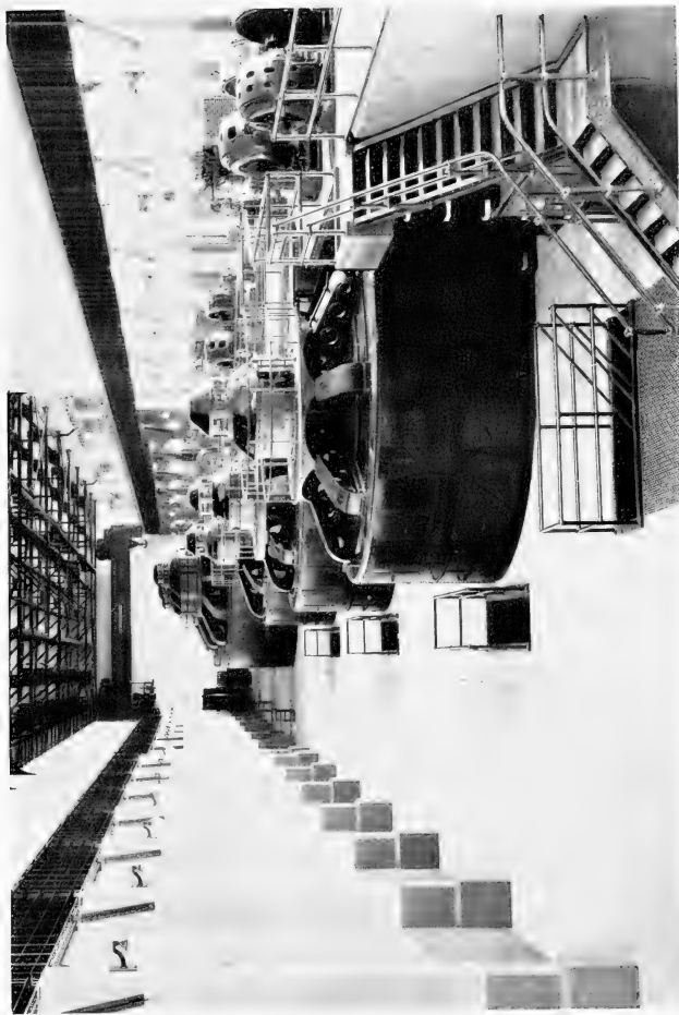
Niagara Falls. Interior of Schoelkopf Station. Three 37,500 h.p. generators in the foreground, three of 70,000 h.p. at the rear. Courtesy of the Niagara Falls Power Company
