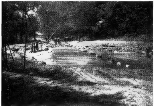
Building the lower ford, view from the east side of the creek, circa 1913.
