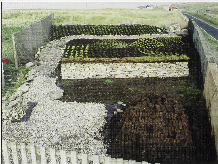
Planting complete – only the vegetable patch and a few finishing touches left to do.
