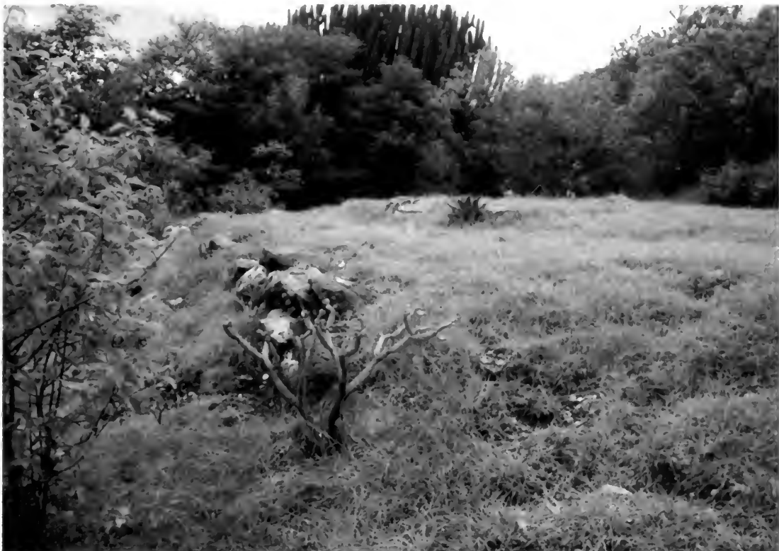
FIG. 5.7. Stone retaining wall and small stone house foundation on Terrace 663 at El Palmillo.
