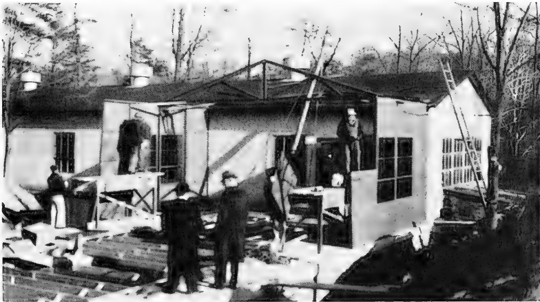
Figure 17. Walls going up on the addition to the BEB's facility on Dalecarlia Reservation, Washington, D.C., winter, 1939-40.
