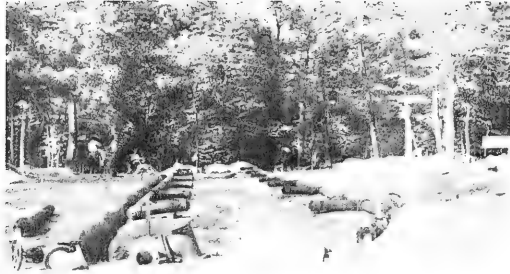
Figure 13. Plumbing for the BEB's 85-foot wave tank on the Dalecarlia Reservation, Washington, D.C., 16 August 1937.
