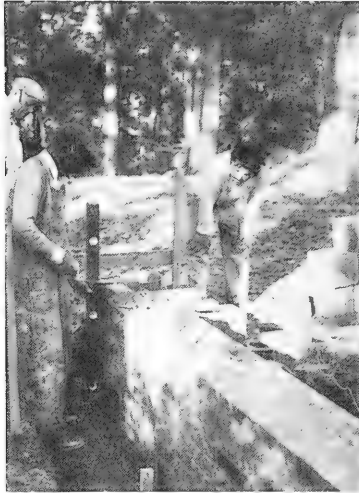
Figure 40. BEB staff workmen preparing foundation for another addition to provide increased office and laboratory space. Left to right: Frank Erwin, Jim Mason, and unidentified.
