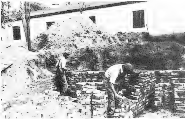
Figure 16. Jim Mason and Frank Erwin laying brick foundation for the first addition to the BEB laboratory building (seen in background). The addition was to provide office space for the Board's staff, 27 October 1939.
