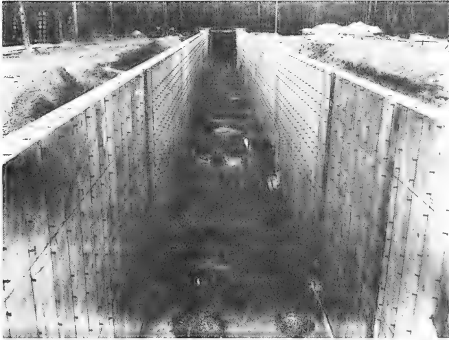
Figure 29. View looking down the 20-foot-deep, 635-foot tank toward area where generator will be located. On the right, shore processes test basin is under construction.
