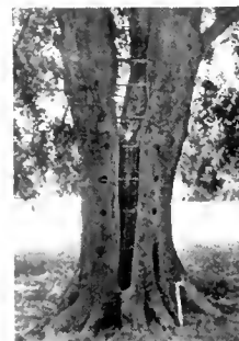
All the decayed matter has been removed and the whole interior carefully disinfected and water-proofed. Mechanical bracing has been employed to strengthen the weakened trunk
