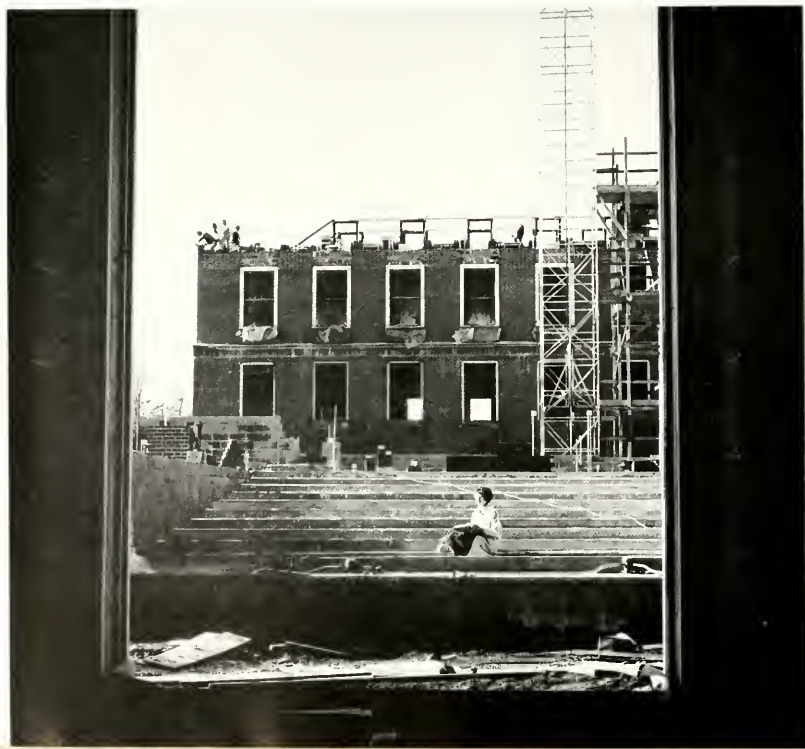
As the building takes shape, a student sitting on the steps of the future auditorium visualizes its eventual use.
