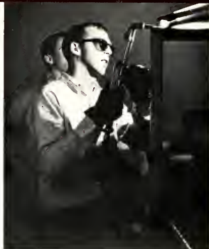
Removing metal trunk storage racks from the walls was only one task in making the Taylor lounge out of a tunnel and storage room.
