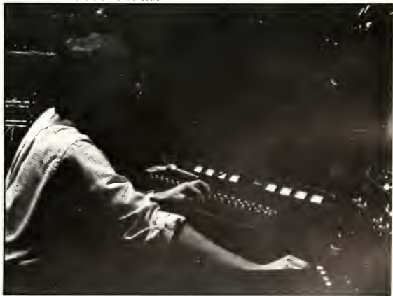
Control board above the main theatre
