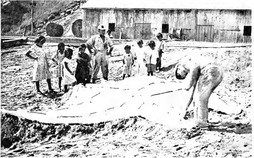
Fig. 171. Ten hours later the last reinforcing rod is attached to the mold.
