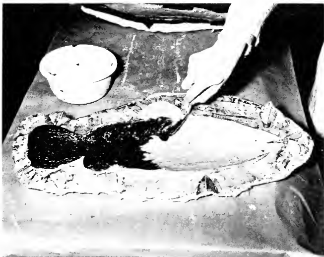
Fig. 55. The second or reinforcing layer is applied after the first coat of plastic has set. This mixture appears black in the photo because it has asbestos mixed in the formula No. 2.
