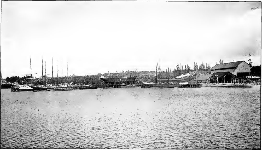
FIG. 17—WOODEN SHIPYARD LOCATED ON NATURALLY SLOPING GROUND WITH AN ABUNDANCE OF ROOM
