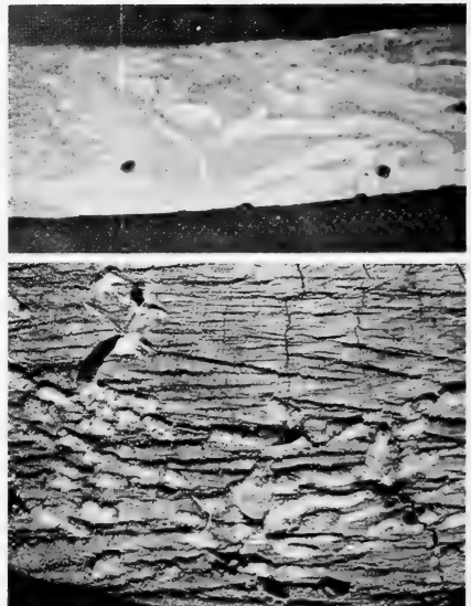
F-504086 FIGURE 80. — Top , tunneling on the wood surface by the red-headed ash borer. (Photo courtesy Illinois Natural History Survey.) Bottom , banded ash borer galleries tightly packed with granular frass.
