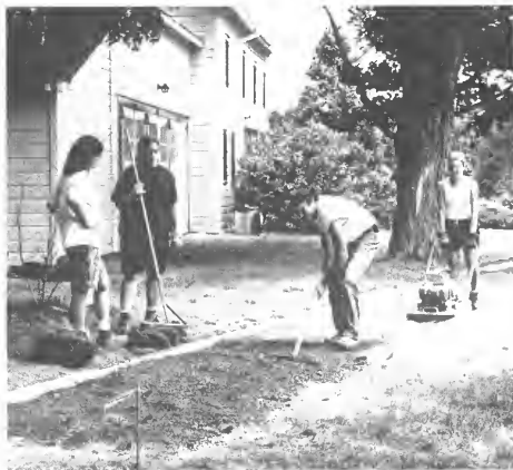
Left: Mr. Brad Roeller and Landmark Volunteers level the new path by the Carriage House.
