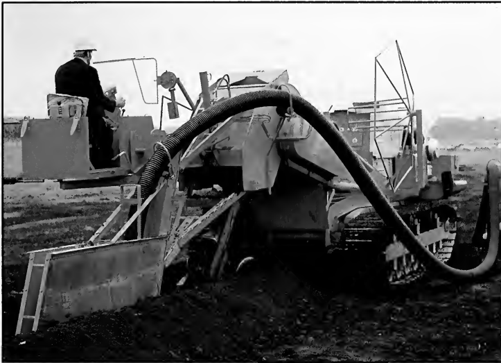
Installing drainage tile. Drainage tile is used extensively in central Illinois to remove excess water from farmland.
