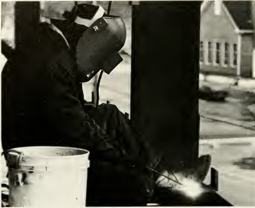
Construction worker Willie Locklear welds on the third floor of the Science Building's new wing. Photo: David Malcolm.
