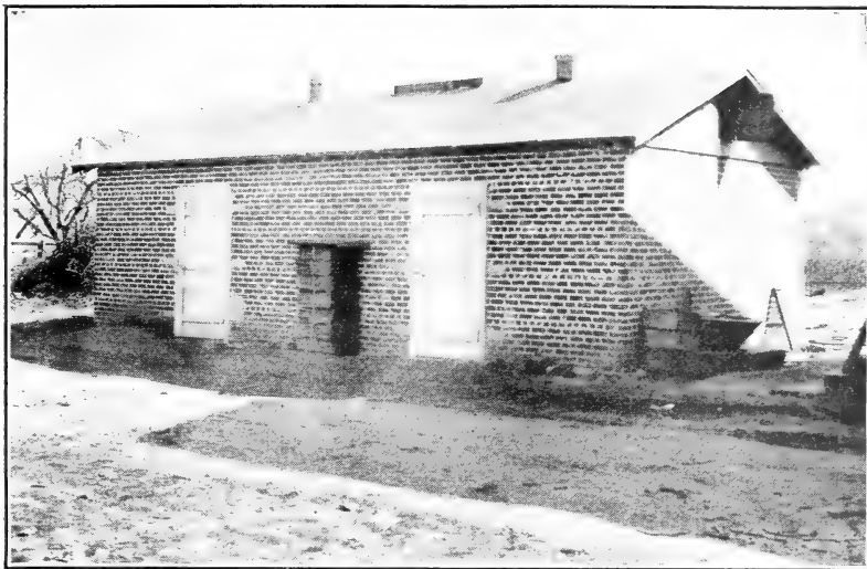
FIGURE 29.—Two outdoor fumigation vaults under one roof, built of brick, finished on the inside with Keen's cement, and equipped with doors shutting against rubber gaskets to prevent gas leakage. Note ventilators in roof to aid in ventilation when lighter-than-air gas is used. (Photograph by Perez Simmons.)
