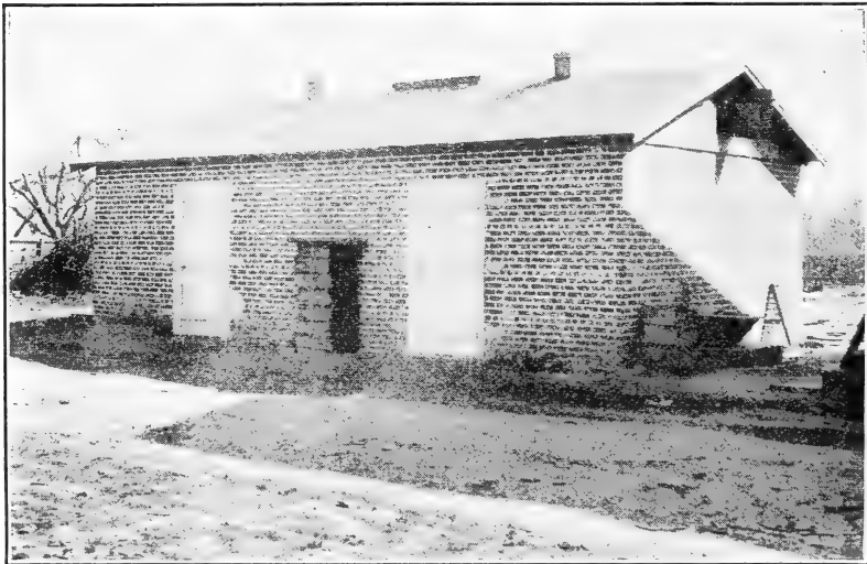
FIGURE 25.—Two outdoor fumigation vaults under one roof, built of brick, finished on the inside with Keen's cement, and equipped with doors shutting against rubber gaskets to prevent gas leakage. Note ventilators in roof to aid in ventilation when lighter-than-air gas is used. (Photograph by Perez Simmons.)
