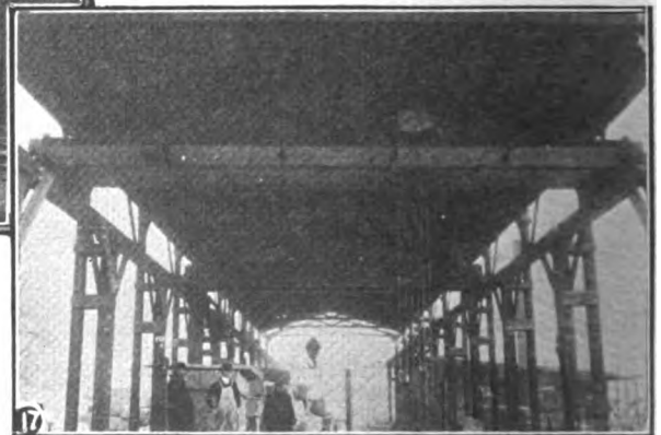
Fig. 17. A roof over the craneway protects machinery and provides a shelter for workmen.
