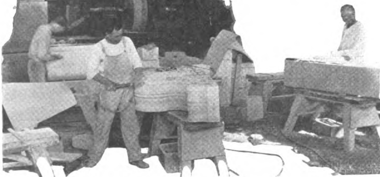
Fig. 3. Placing a huge building column in front of a bank building in New Orleans.
