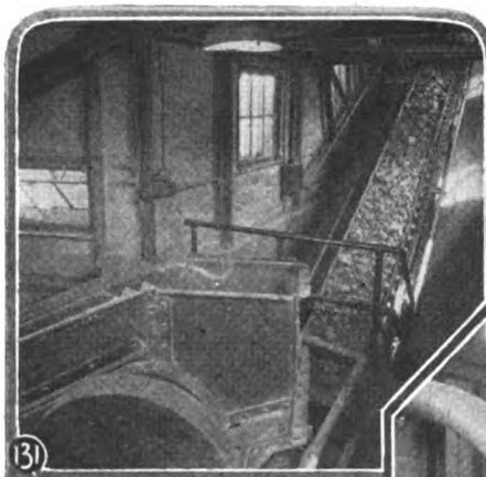
Fig. 131. Lump slag is taken from the track hopper by a beaded flight feeder and conveyor.
