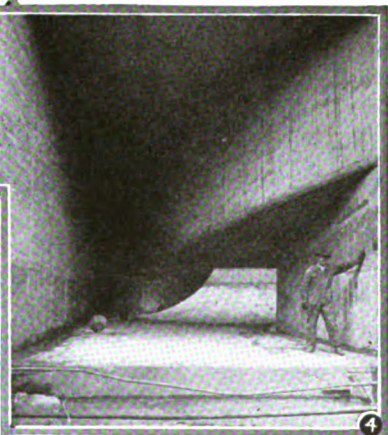
Fig. 4. Draft tube section of a turbine setting, showing the water's path after leaving the turbine.
