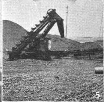
4—The Barber-Greene which unloads a 50-ton car of Shamrock 4-inch lump in 59 minutes. It has eliminated storage bins near the tracks, and has increased the storage capacity of a limited area.
