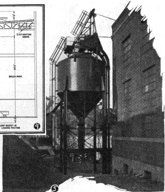
Fig. 5. Actual installation of equipment, shown in Fig. 4. This installation is of a semi-automatic skip hoist and storage bin for ashes installed at the Steele Lighting Plant, City of Jamestown, N. Y.
