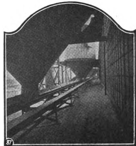
Fig. 87. Close-up view, showing connection between cyclone collectors and cable flight conveyor which transports the refuse away.
