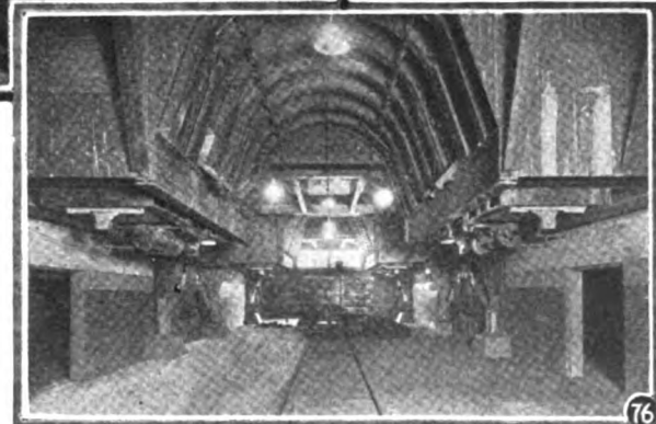
Fig. 76. The efficiency of this boiler house and power plant is such that very little ash or cinder needs to be drawn off from the boilers. For this reason no conveyor system is installed.
