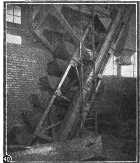
Fig. 40. General view of one of the new perforated bucket elevators for the handling of granulated slag.
