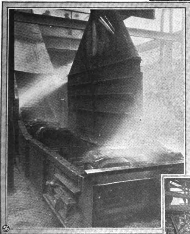
Fig. 56. Loading station of a hot casting conveyor which elevates the hot castings to the mezzanine or cooling floor.
