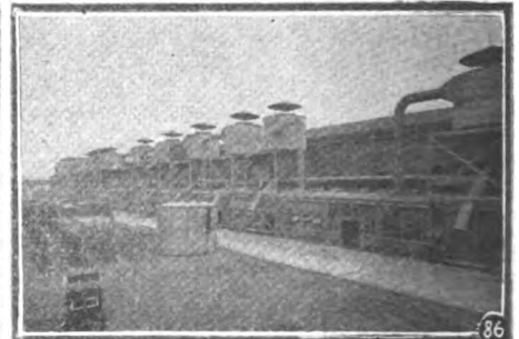
Fig. 86. Battery of cyclone collectors, which are part of the pneumatic conveying system.
