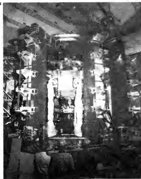
7 Cleanliness within the vacuum vessel is essential for successful machine operation. To achieve this the metal vessel is of a welded construction and can be baked to 500°C to remove surface impurities. Each section of the vessel is made from five rigid units joined by sets of flexible bellows. The bellows increase the electrical resistance of the chamber so that the current flows mainly in the plasma rather than through the vessel.
