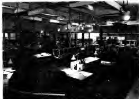
Computer and control rooms
