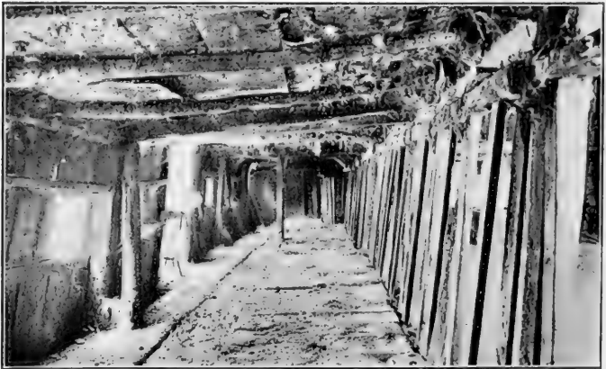
TIE-UP WITH DIRTY, DEFECTIVE FLOOR, CEILING, AND BACK.
