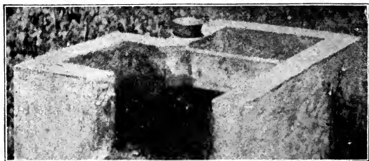
Fig. 64. Same hydrant as Fig. 63, with water discharging over left wier into underground pipe.
