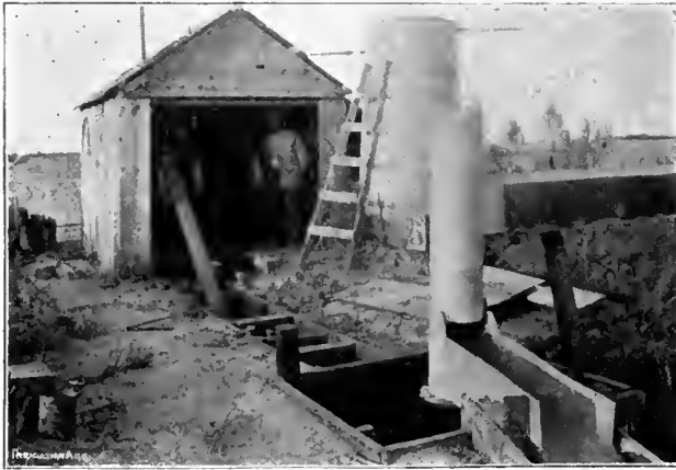
PUMPING PLANT OF R. W. BRISCOE, Near Malaga, Cal.
