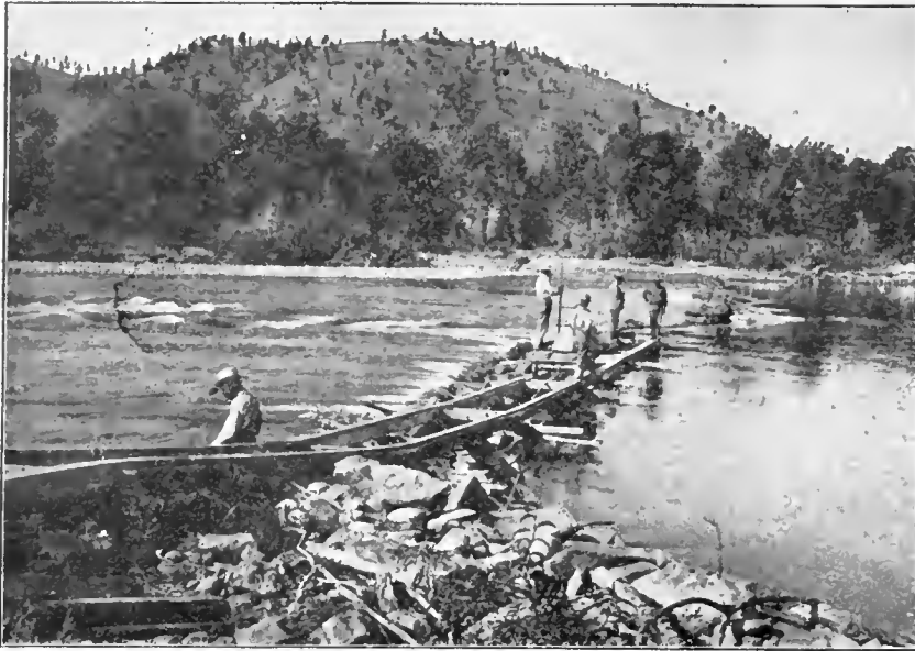
Courtesy U. S. Dept. Agriculture. (Mead.) IRRIGATION INVESTIGATIONS—REPAIRING BRUSH AND ROCK DAM, YELLOWSTONE RIVER, MONTANA.
