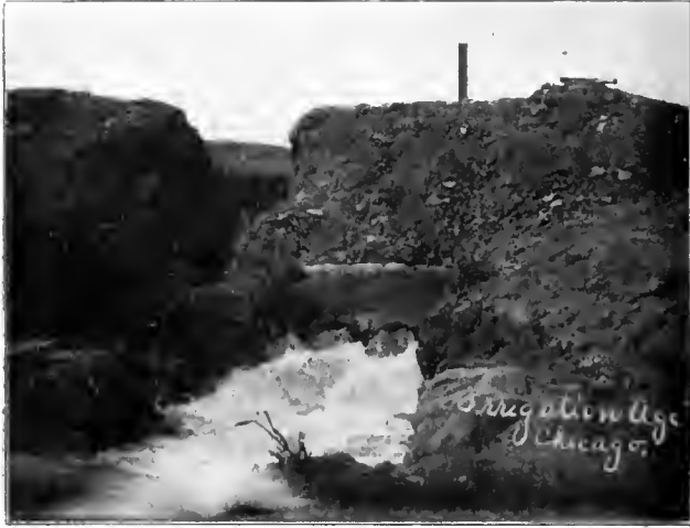
Concrete Outlet from Main Canal of Billings Land and Irrigation Co.'s Canal which forms Lateral shown in another view
