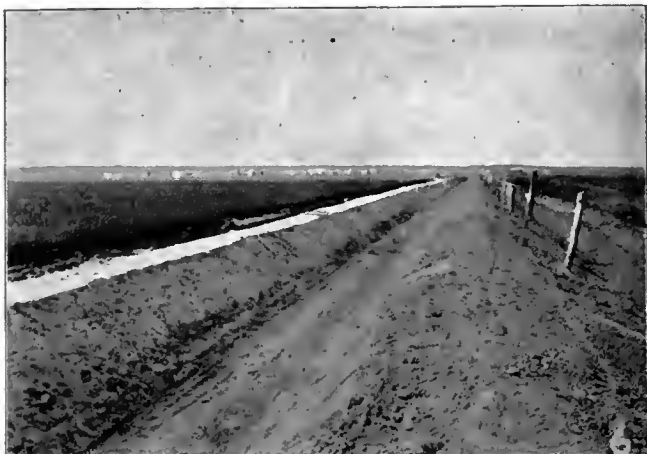
Partly finished lateral, with new town of Sidney, Mont., in the distance.
