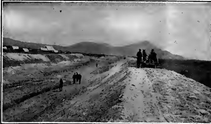
Digging the Main Canal of the Klamath Project; More Than 100 Miles of Main Canal Will Be Required.
