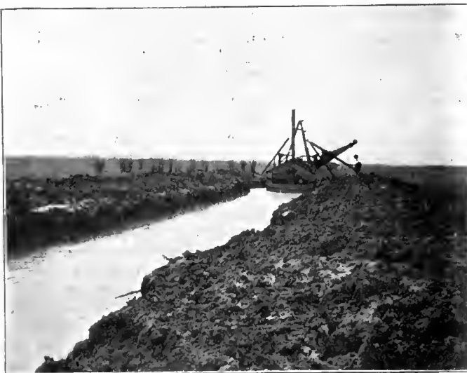
View of a dipper dredge in operation, showing the vertical banks and waste bank constructed immediately adjoining ditch.
