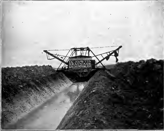
Rear view of Austin Drainage Excavator, showing perfect slope of banks and wide, clean berms.
