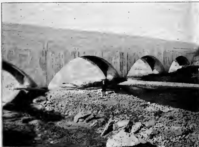
Concrete Flume across Pecos river. Main view, December 18, 1905. Carlsbad, N. M., Project.
