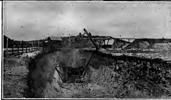
Excavating a Tunnel in the Klamath Project; One of the Expensive Details of the Undertaking.
