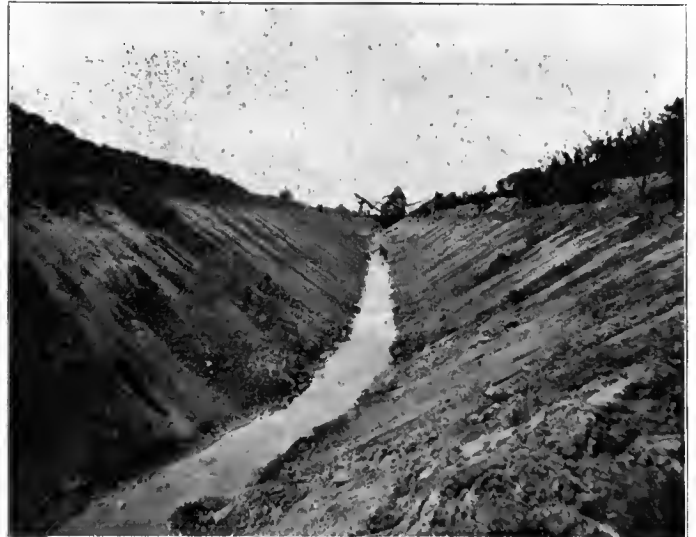
Ditch 12 feet deep, with 4-foot bottom and 1\frac{1}{2} to 1 slope built by the Austin Drainage Excavator in Cass County, Ind., illustrating ditch that is perfectly self-cleaning where there is a variable flow of water.
