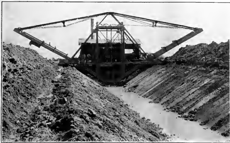
Improved Type A Machine digging ditch with 8 ft. bottom, 1\frac{1}{2} to 1 slopes, 10 ft. deep, 8 ft. berm.
