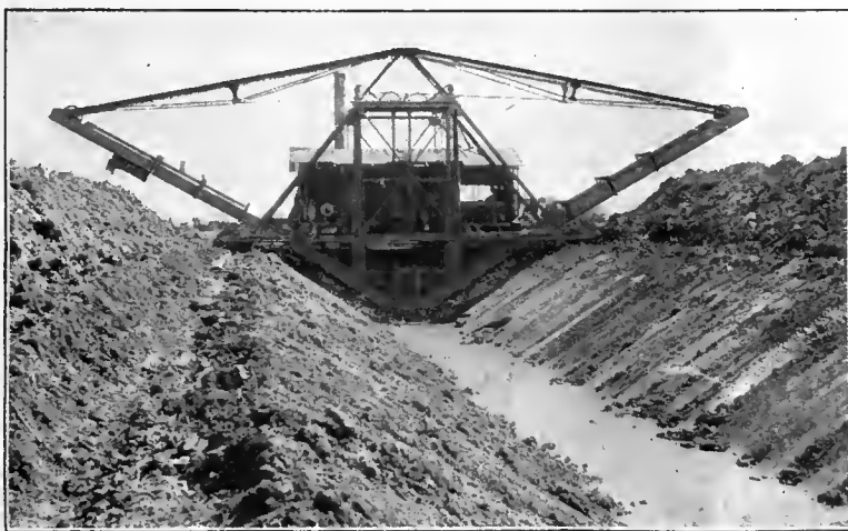
Improved Type A machine digging ditch with 8 foot bottom, 1\frac{1}{2} to 1 slopes, 10 feet deep, with beam of 8 feet
