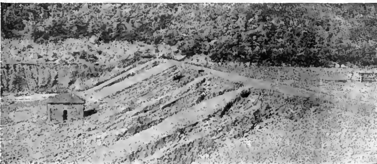
FIGURE 3. Earth Dam at Altoona, Pa., showing effect of wash.
