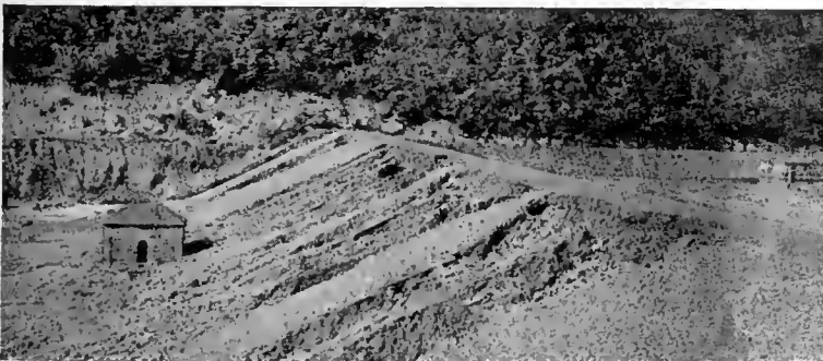
Fig. 6. Altoona Dam, Showing Incipient Failure From Wave Spill.
