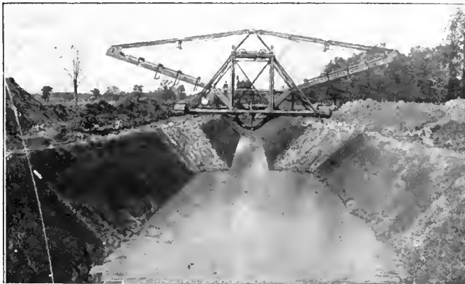
Ditch Being Dug with Sloping Banks—An Austin Drainage Excavator Ditch, showing variations in width made with same machine
