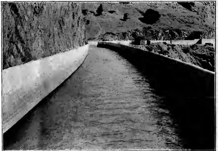
CONCRETE IN IRRIGATION CANAL CONSTRUCTION Concrete-Lined Main Canal of the Modesto Irrigation District, California
