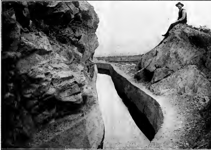
Okanogan Project, Washington. Concrete-lined Canal Section, Partly in Rock Cut, at Pogue Flat.
