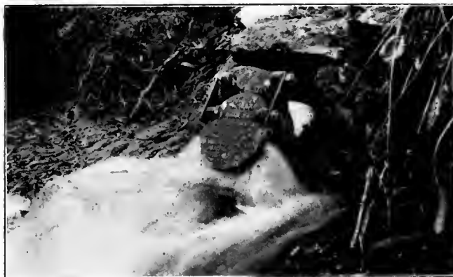
Close-Up View of 8-in. Calco Auto-Drainage Gate Discharging Storm Water From Gutter Into Irrigation Canal (P. 136).
