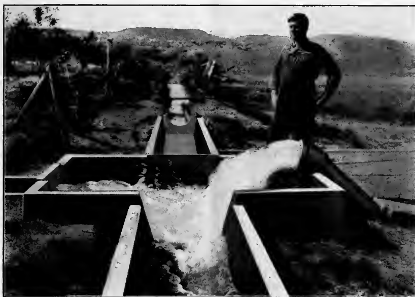
Four-way Distributing Box of Concrete, Receiving Discharge From Artesian Well, El Paso, Texas.
