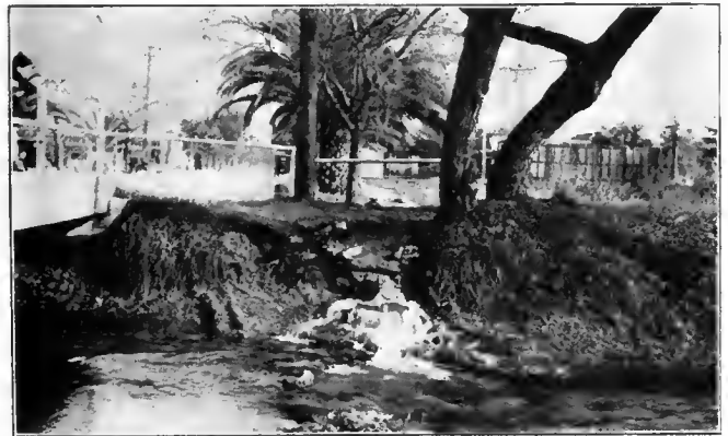
30-in. Calco Auto-Drainage Gate in Operation Discharging Water from Gutter Into Irrigation Canal in City of Fresno, Calif.
