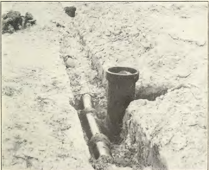
FIG. 2.—WATER-TIGHT MAIN AND STOP-BOX CONNECTION TO SUBIRRIGATION LATERALS, SANFORD, FLA.
