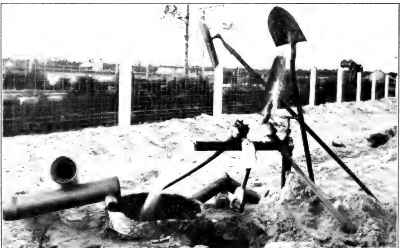
FIG. 3.—WATER SUPPLY AND TOOLS USED FOR SUBIRRIGATION, SANFORD, FLA.
