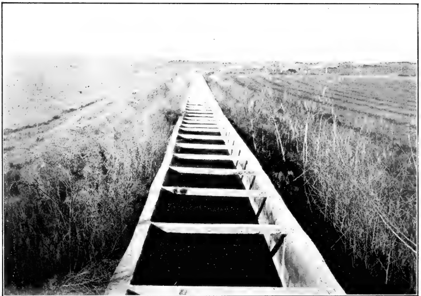
FIG. 2.—FLUME OR CHUTE CARRYING LONG POND WATER TO THE LARIMER AND WELD CANAL AND LINDENMEIER LAKE.
