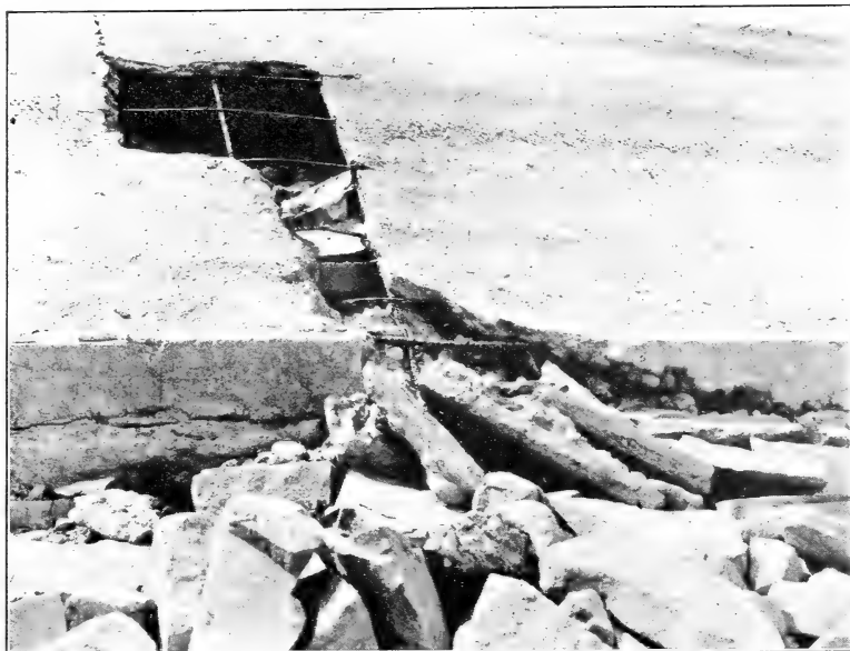
FIG. 1.—CLOSE VIEW OF BREAK IN THE PAVEMENT OF TERRY LAKE.
