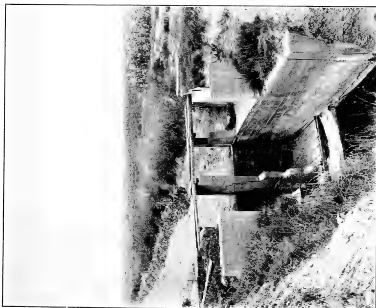
FIG. 1.—CONCRETE DROP ON THE INLET TO THE COAL CREEK RESERVOIR OF THE NORTH POUDDRE IRRIGATION Co.
