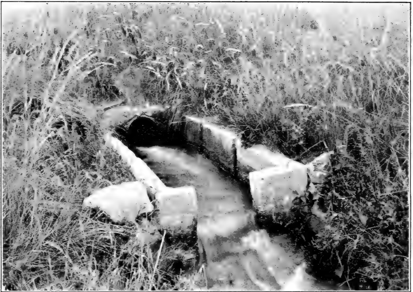
FIG. 1.—DEVICE FOR MEASURING WATER DELIVERED TO THE LATERALS OF THE PLEASANT VALLEY CANAL.
