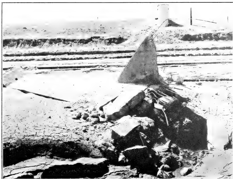
FIG. 2.—GATE TOWER BLASTED OUT AND REPLACED BY A WELL WITHIN THE DAM. NORTH POUDBRE RESERVOIR NO. 15.
