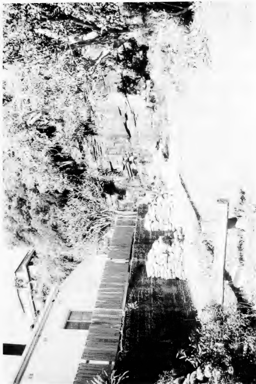
21. Protective measure adopted below a major waterfall on flood path (Dover Road). The supporting wall of this house suffered considerable damage.
