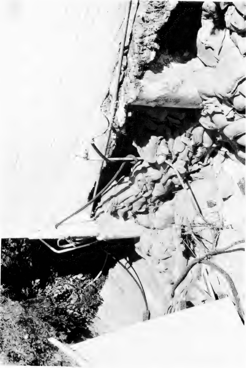
14. Undercutting along College Lane by sand-laden water from pipe outburst.
