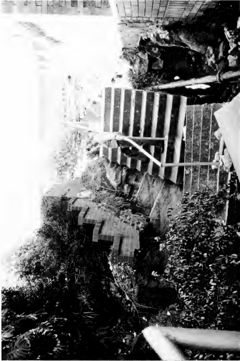
20. Collapse of structures built immediately over sandstone along a major flood path (off Liverpool St.).
