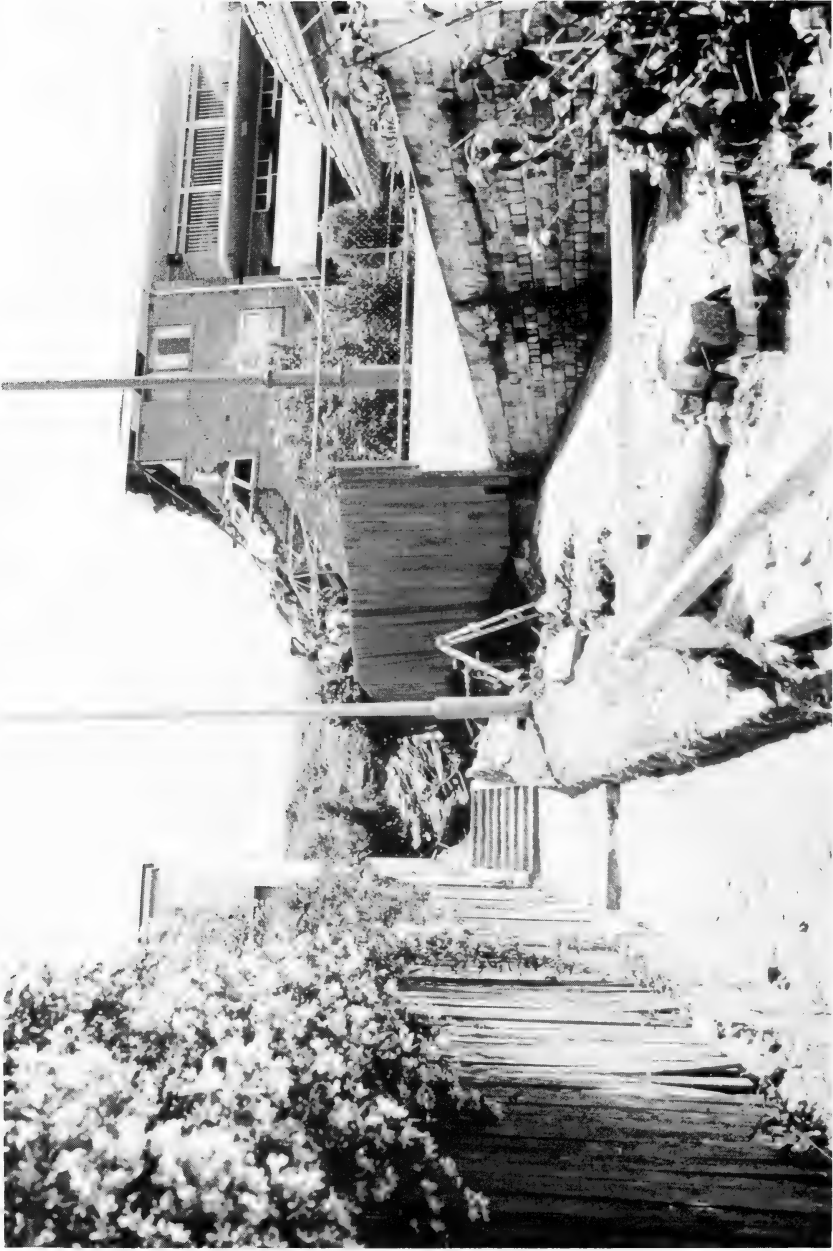
15. View up College Lane to Scots Oval. Note narrow, straight, stepped flood course. Concrete along left side of path has been severely eroded.
