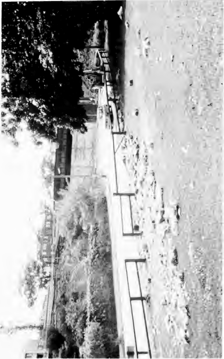
4. Coarse debris in Waverton Park carried from slumped embankment in right background.
