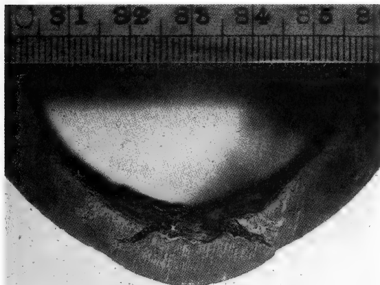
Fig. 2. Part-section through high-pressure boiler tube corroded from the inside almost to failure. The two radial fissures mark the extent of cracking of embrittled metal, but the outside of the tube has remained ductile and bulged rather than cracked.
