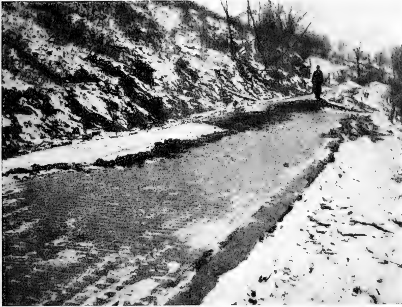
FIG. 5.—Slides have undermined the brick-paved road at this point. The line of dirt through the center of the road fills a crack and reduces the gradient between the sides of the offset. At the far end marked by the position of the man, half the road has dropped to such an extent as to require blocking off.
