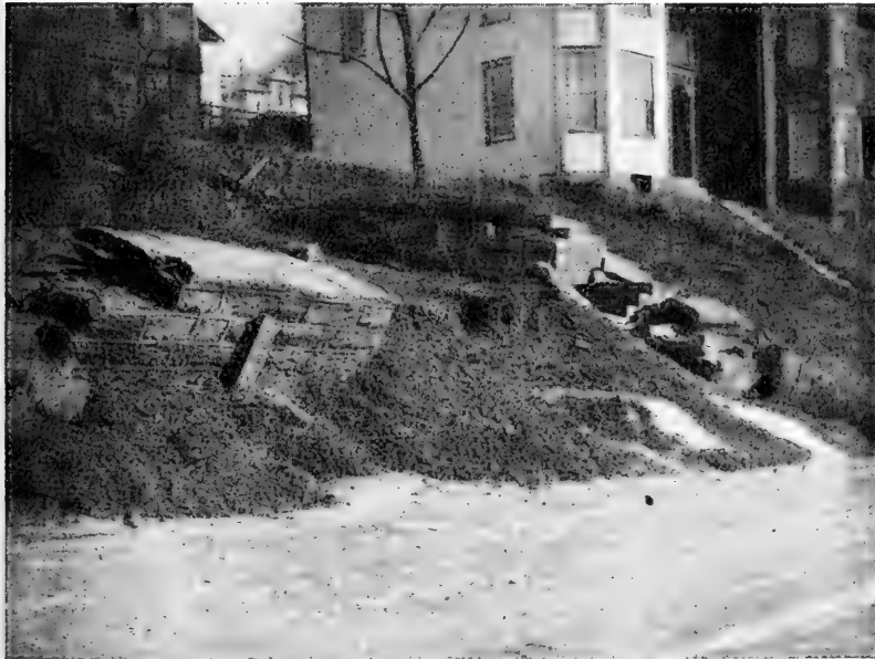
FIG. 3.—Walls and steps pushed forward as a result of slide movements. The house in the foreground is in immediate danger. Note jagged edge of broken brick walk leading to house in the rear. As is frequently the case, the sliding masses have produced a terrace-like form, with the vegetation growing on its top but little disturbed. Many months were required to produce the foregoing result.
