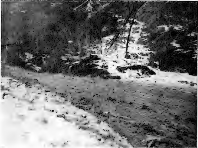
FIG. 4.—Slide partially blocking roadway. The entire face of the slope above the slide is bare to a height of about forty feet, the result of recent slides.
