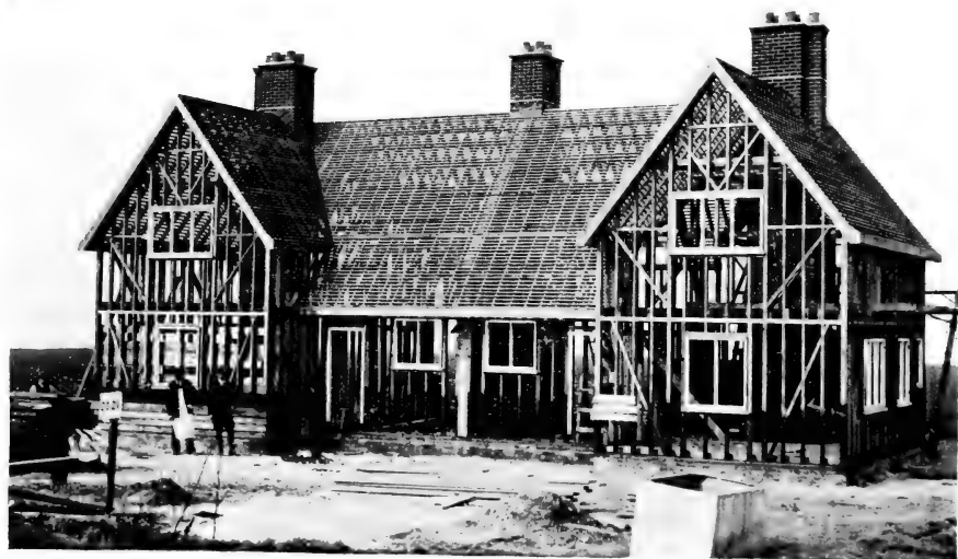
FIG. 6.—Timber Cottages. View showing framing ready for weather boarding and roof tiling.
