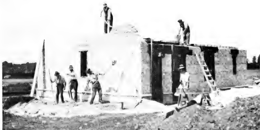
FIG. 2.—Chalk Cob. Chalk walling in process of erection. Traditional method. Also showing concrete lintels cast in situ .
