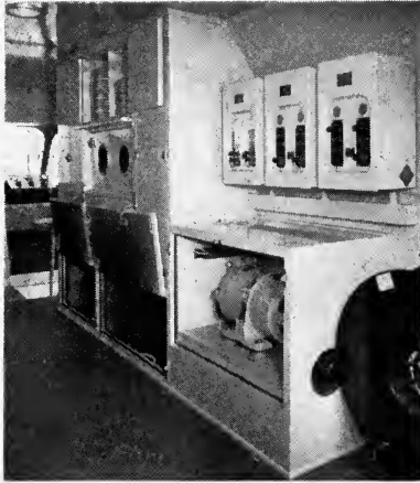
FIG. 5. Power batteries are serviced through compartment doors at left. Motor generator set is shown at right.
