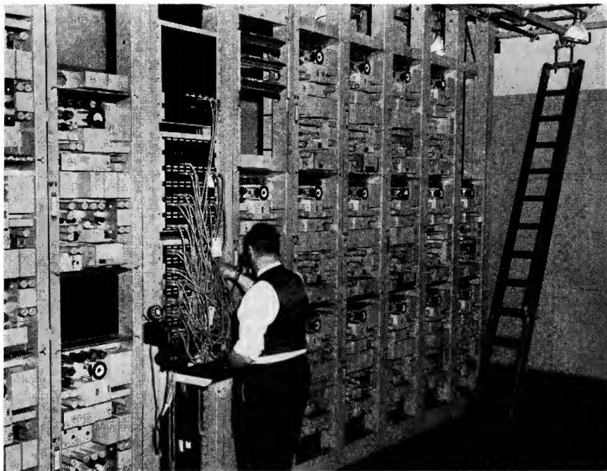
Fig. 5. Video amplifiers in telephone central office.
