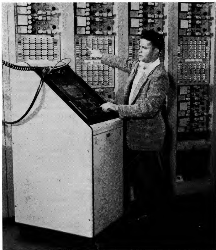
Fig. 8. Intercity video pushbutton switching panels.
