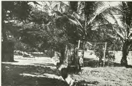
FIG. 3.—Completed concrete drain put in after settling down has finished and permanent level reached.
