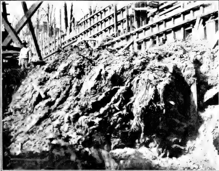
Fig. 5. Portion of a stump and roots still in place in the swamp muck on the north side of the excavation.
