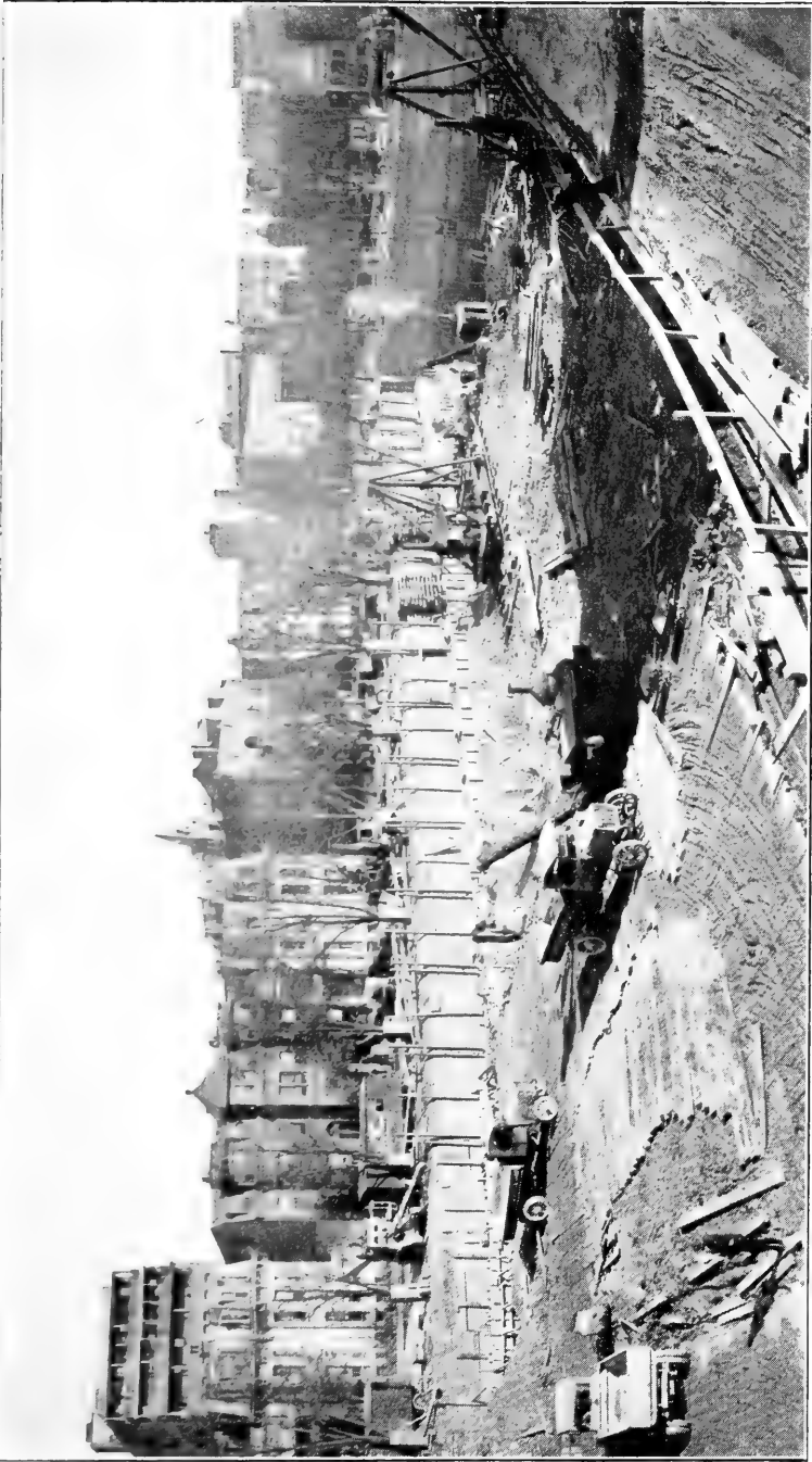
Fig. 2. General view of the east end of the Walker Hotel excavation. The steam shovel near the northeast corner is engaged in removing the materials of the Pleistocene swamp deposit, the top of which lies just below the level on which the hoisting machinery stands. Photograph reproduced by courtesy of the Walker Hotel Organization.
