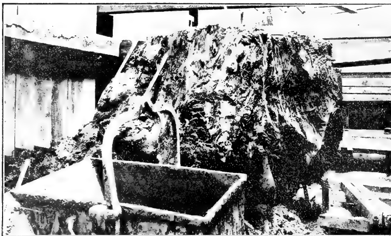
Fig. 3. One of the larger cypress stumps still in place but exposed and portions of it cut away in the process of digging. Sheet piling and one of the loading buckets are also prominent in the picture.
