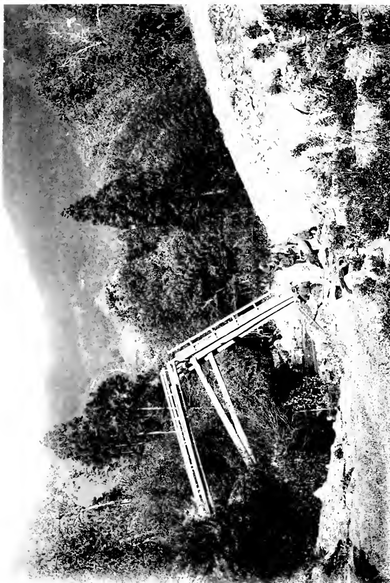
RUINED BRIDGE IN THE NÉO VALLEY.
