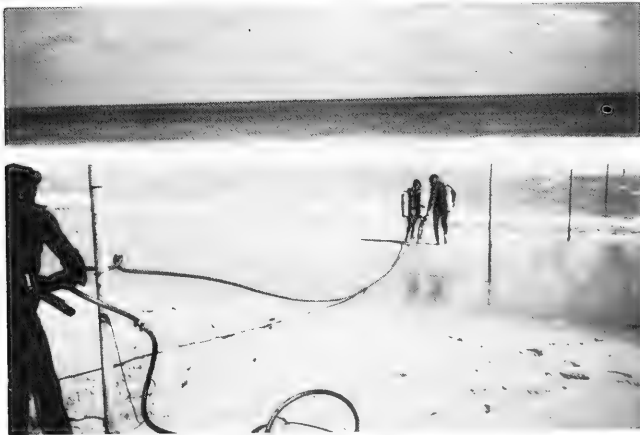
Figure 16. Pneumatic jackhammer setup for driving profile pipes into sand and beach rock.
