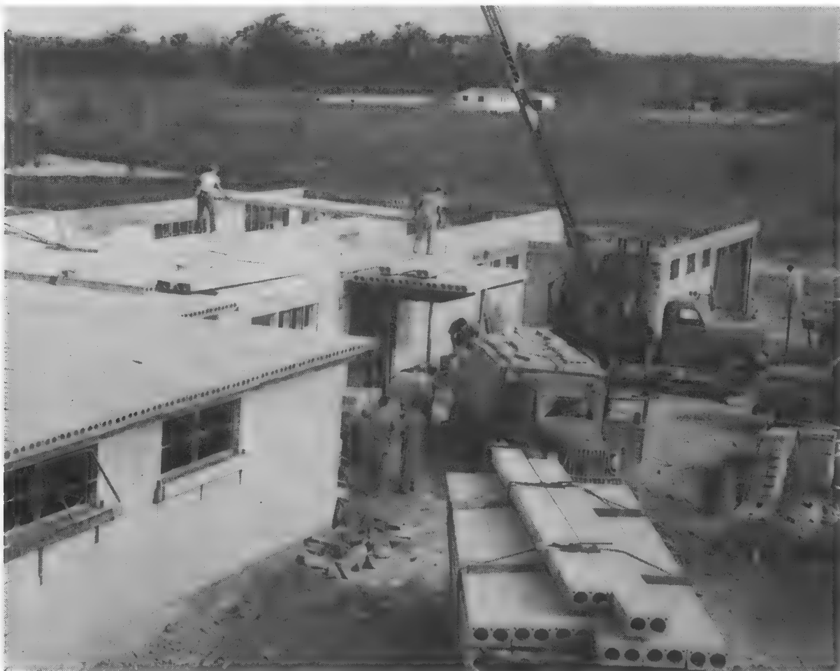
Below , the Laboratory building 2 August 1956. The roof is being laid with flexicore slabs. Photographs by David G. Allen.
