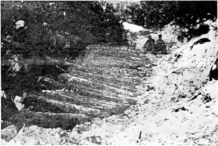
FIG. 44. — A Two-sled Road, showing the Method of building up the Grade on Slide Slopes.
