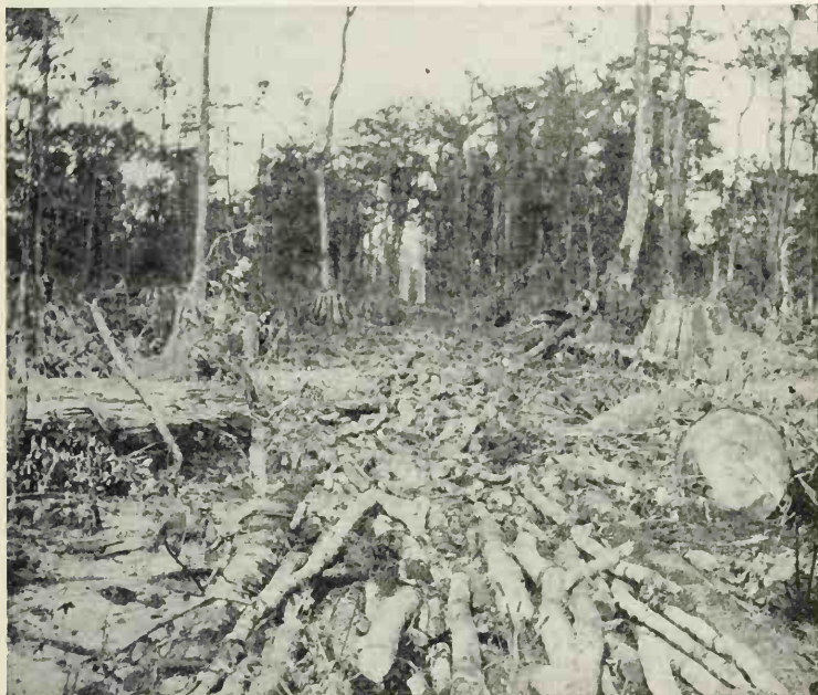
FIG. 103. — The Pole Foundation for a Dunnage Road in a Cypress Swamp, Louisiana.
