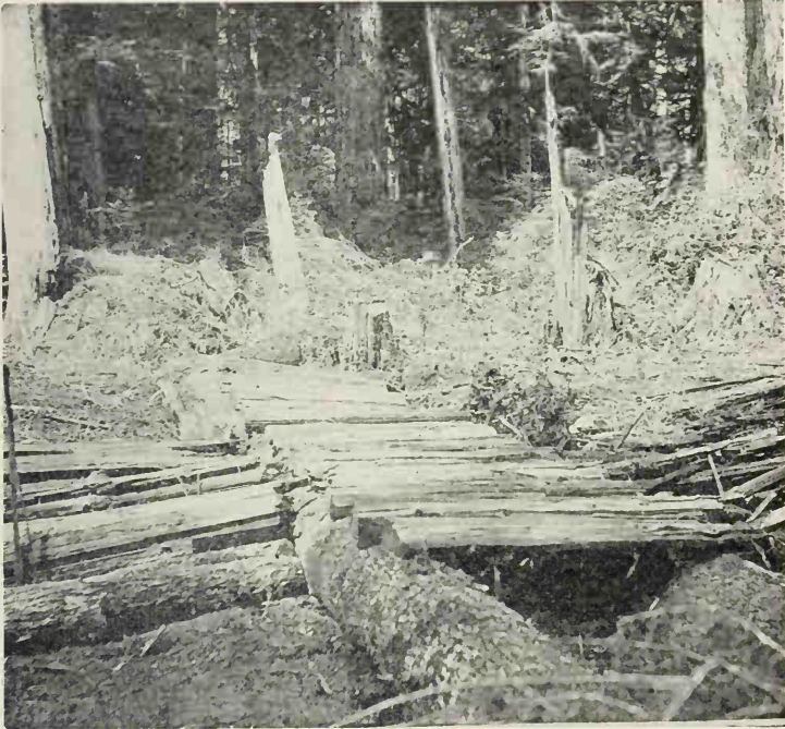
FIG. 106. — A Culvert on a Logging Railroad Spur ready for the Earth Cover. Note the use of non-merchantable material for filling depressions on both sides of the culvert. Washington.
