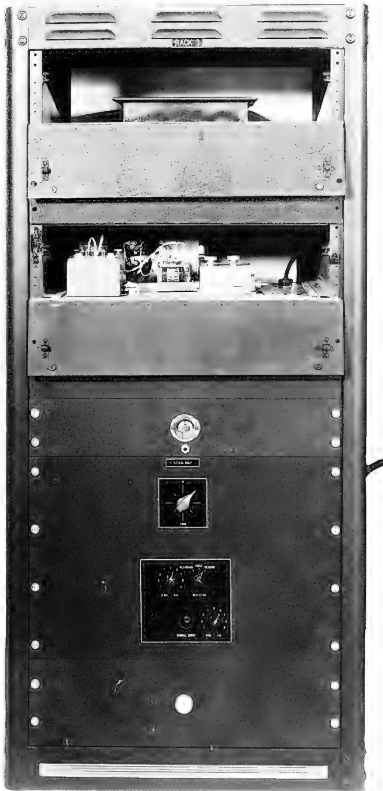
FIG. 9 - Rack Three, Front View
