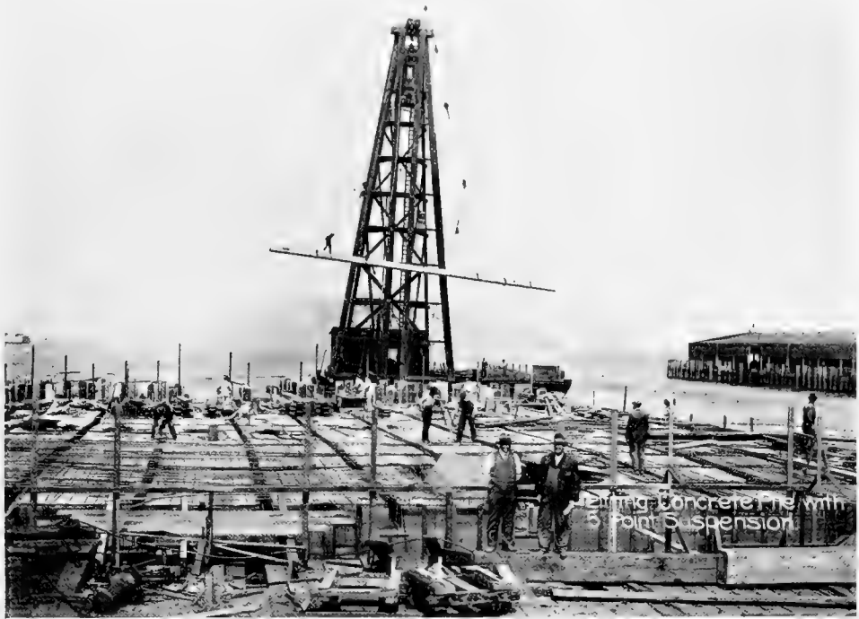
Fig. 51. Handling 105-foot concrete pile with 5-point suspension, Pier 3, San Francisco. (Board of State Harbor Com's. Photo.)
