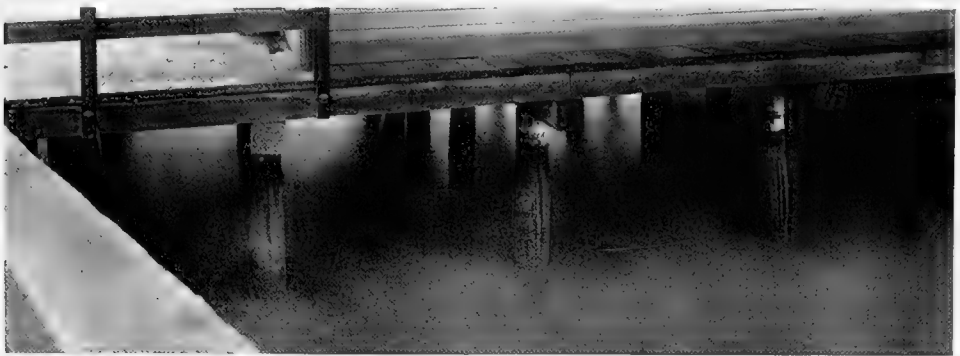
Fig. 38. Bulging battens on piling protected by Moran and Paraffine processes at Georgia St. wharf, Vallejo, after three years' service. (S. P. Co. Photo.)
