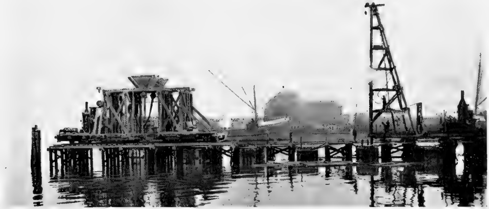
Fig. 52. China Basin Terminal San Francisco. Concrete caisson construction, showing tops of caissons in place, piles being driven inside caissons and concrete being poured. (Board of State Harbor Com's. Photo.)
