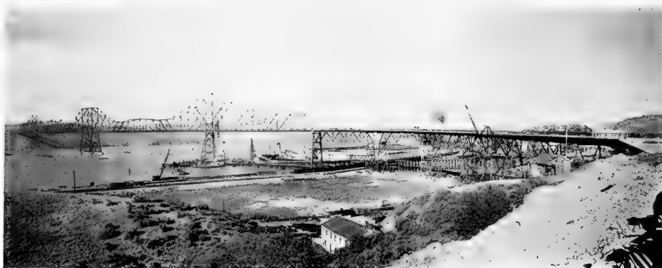
Fig. 16. Carquinez Bridge during construction. California and Hawaiian Sugar Co. plant (location of test station C) is behind approach at right side.
