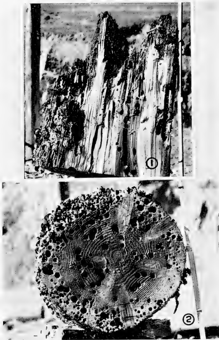
Fig. 32. (1) Dolphin pile from Richmond Municipal Pier, driven December, 1917, broken out July, 1920. Note large tubes of Bankia and smaller ones of Teredo navalis , and erosion by Limnoria at breaking level. Sphaeroma also present. Breaking zone exposed at low tide. (2) Section of same pile, one foot above break.
