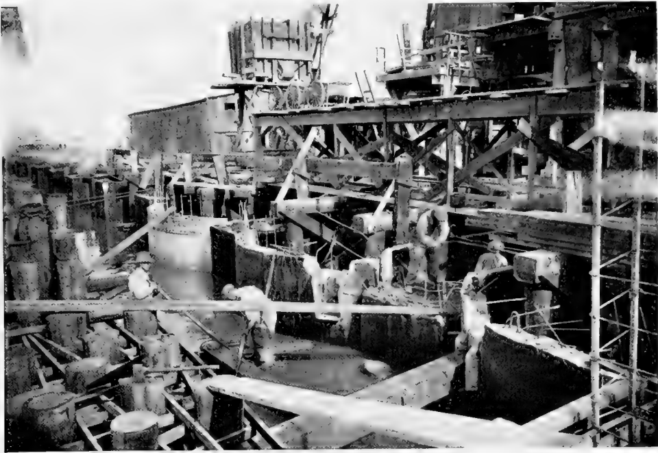
Fig. 15. China Basin terminal during construction, showing caissons after filling (workman whose hands are blurred is standing in one) and pre-cast curved arch slabs in place. (Board of State Harbor Coms. Photo.)
