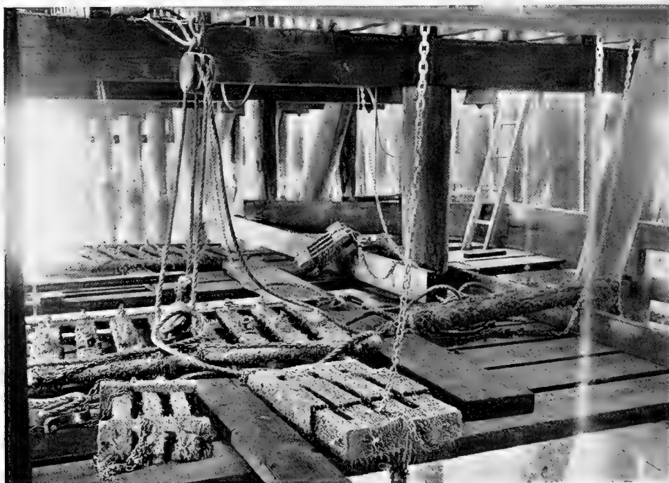
Fig. 3. Test station A at Oakland Mole, showing the high tide level platform underneath the wharf, with several test gates pulled up for inspection.
