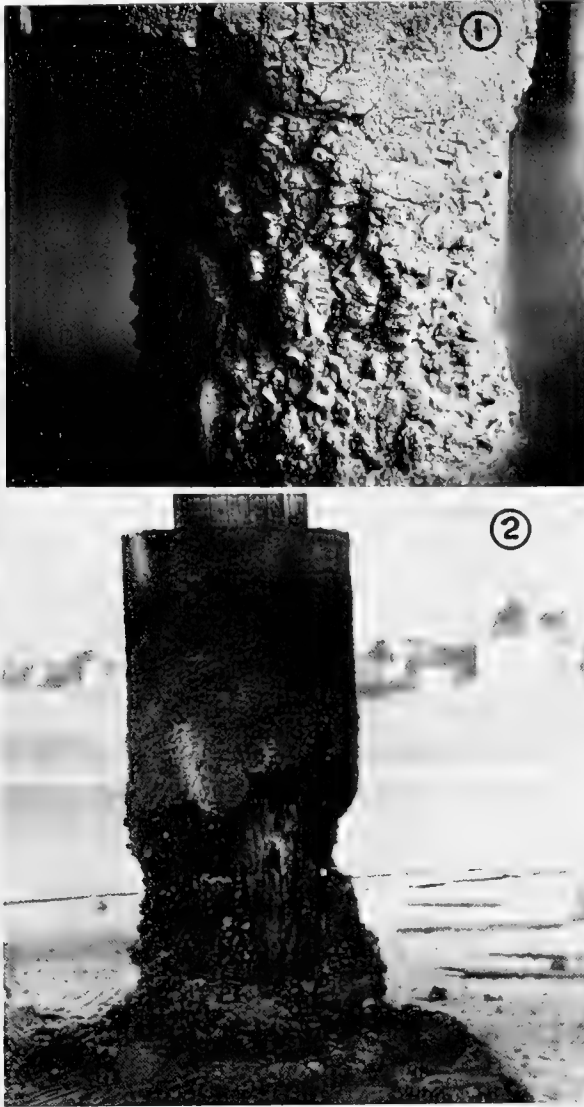
Fig. 29. (1) Disintegration in concrete composite pile. Probably a result of poor workmanship. (2) Disintegration in concrete jacket placed on pile previously covered by battens and paint. Pile attacked by Limnoria where coverings have failed.
