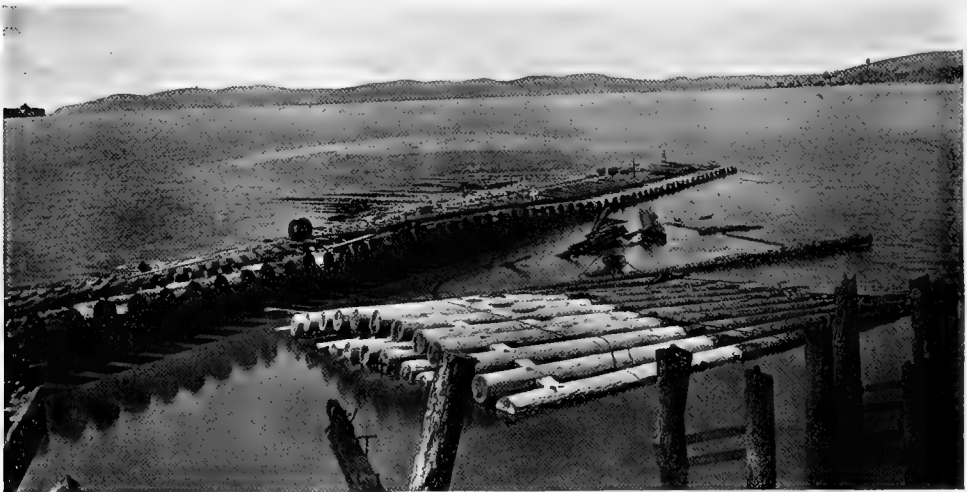
Fig. 14. Untreated ferry slip fender piles in Carquinez Strait, destroyed by Teredo in 1919. (S. P. Co. Photo.)
