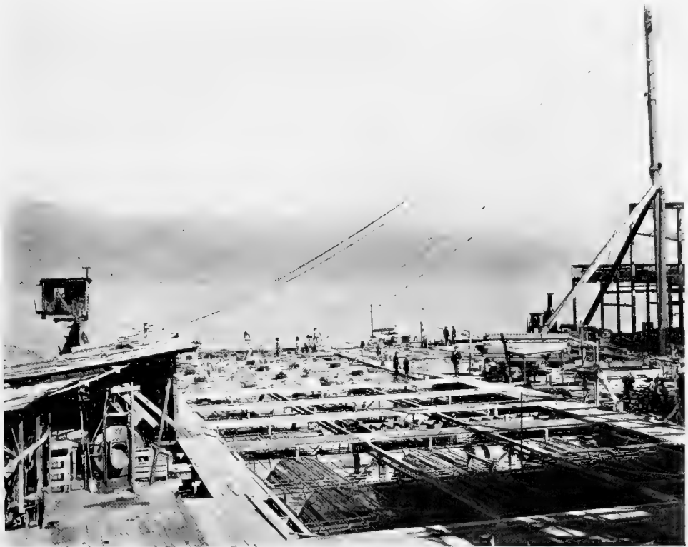
Fig. 53. Construction of California-Hawaiian Sugar Refining Co. warehouse at Crockett, showing tops of reinforced concrete piers and forms in place for groined arches.
