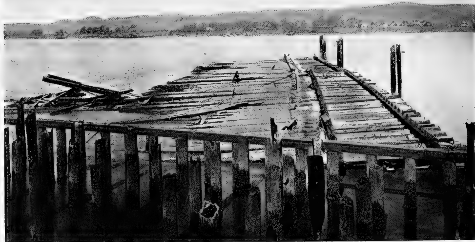
Fig. 12. Untreated ferry slip fender piles in Carquinez Strait destroyed by teredo, 1919. (S. P. Co. Photo.)
