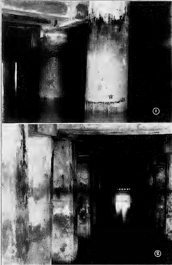
Fig. 59. (1) Reinforced concrete cylinders, Pier 28, San Francisco. Disintegration of concrete due to poor workmanship and improper tamping. These cylinders were repaired by encasing in dense concrete. (2) Reinforced concrete piles, Pier 35, San Francisco; 6 years exposure, excellent condition.
