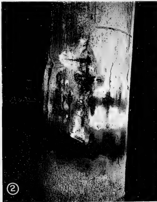
Fig. 48. Concrete jacketed pile, pre-cast type, showing typical rusting crack above high tide level. From bulkhead between Piers 28 and 30, San Francisco; driven 1909.
